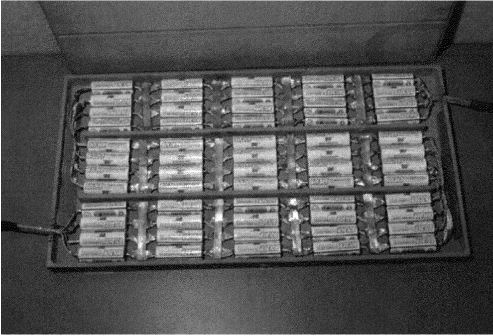
Fig. 15. Single tray of 300 V / 4.8 Ah prototype battery used in Dodge intrepid ESX.
